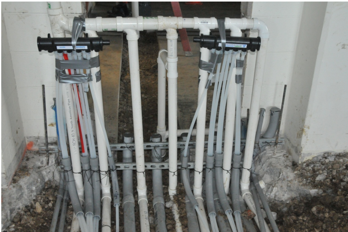
Stoltz Room 9 water/sewer/gas manifolds
